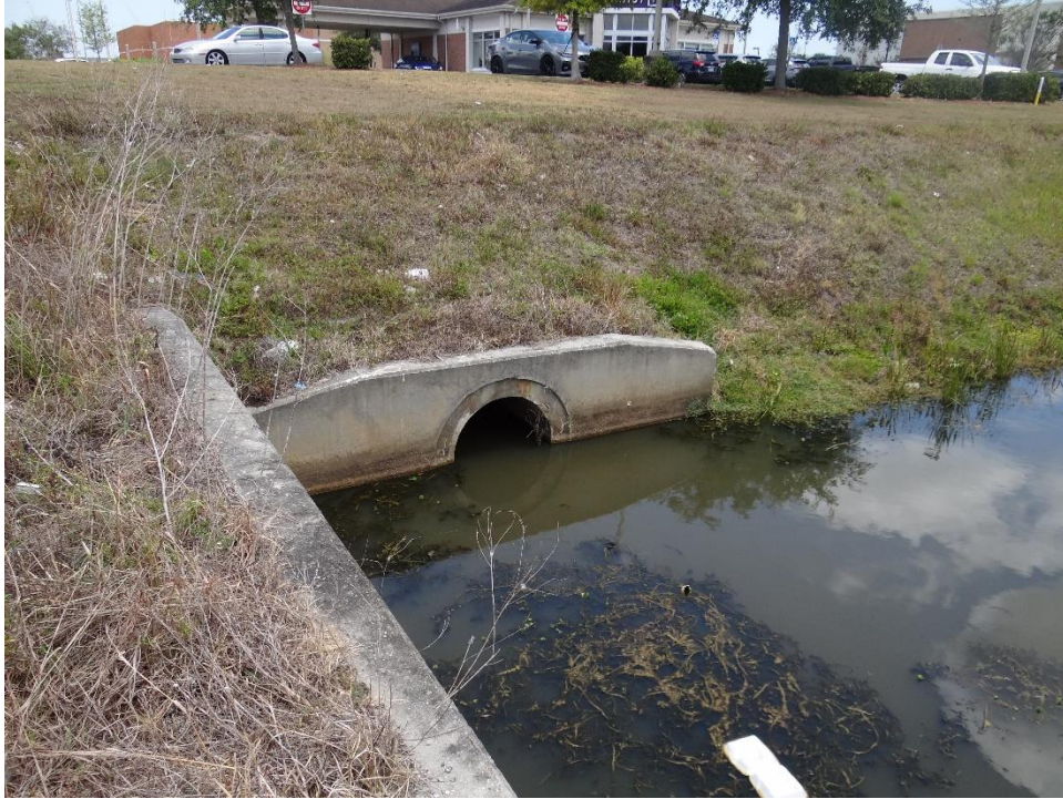
POND A OUTFALL PIPE
