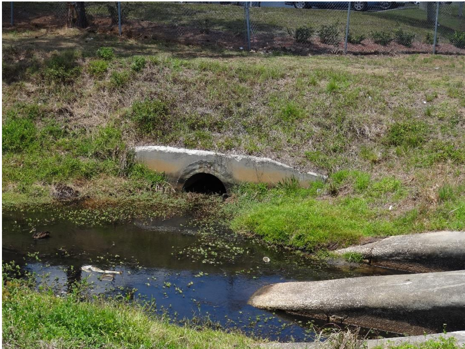
POND B OUTFALL PIPE
